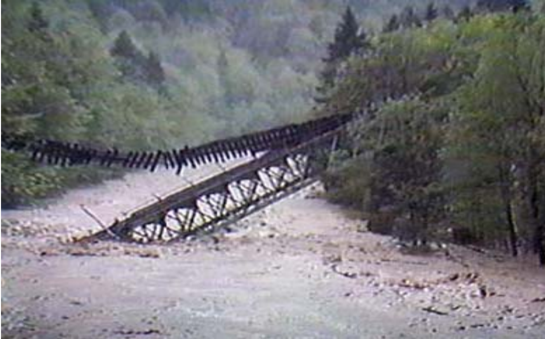
Figure 4: Damage to access bridge caused by flooding.
